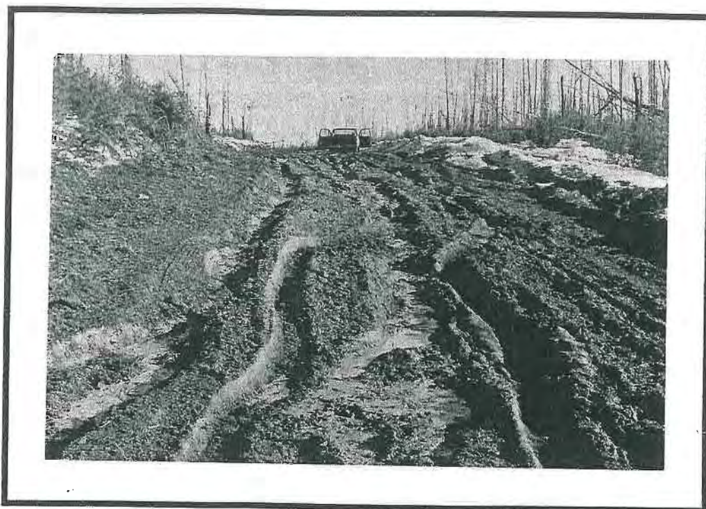
Severe Damage Manifested In Rutting, Concentration of Meltwater, Erosion and Sedimentation Results From Using Winter Roads Too Late Into The Spring.
