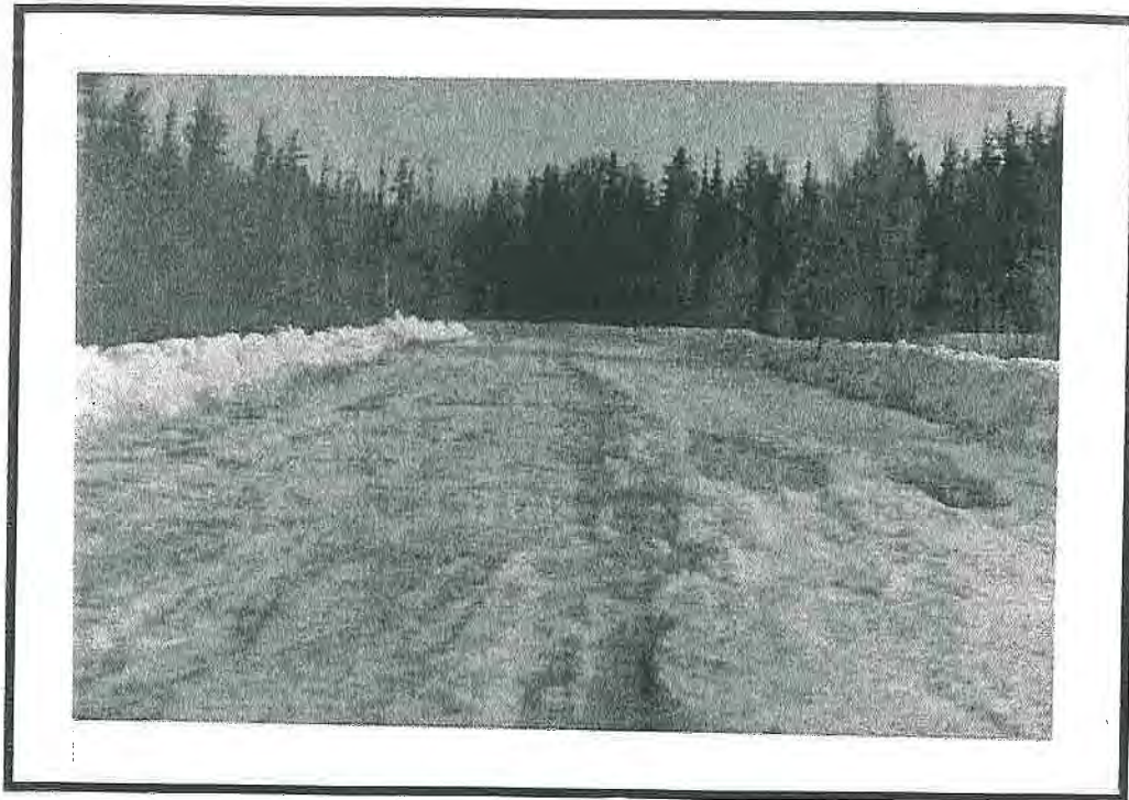
Once Temperatures Approach 0°C Increased Inspection Is Necessary To Avoid Terrain Damage or Damage To The Road.
