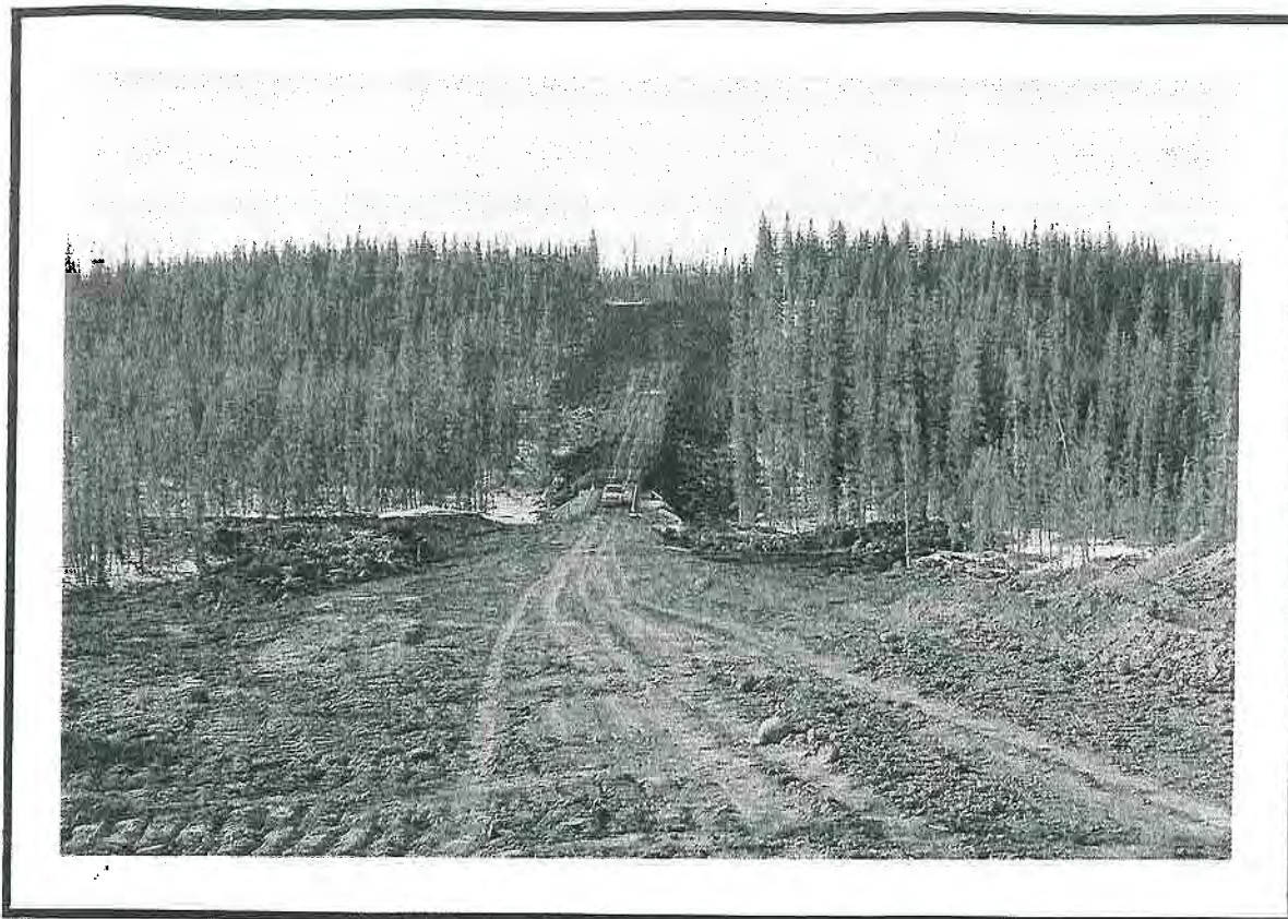
Major Work Such As Cutting Back Slopes At Creeks Should be Preceded By An Extensive Drilling Program
