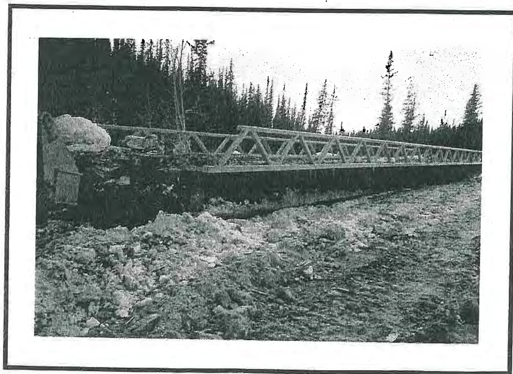
Removal Of Temporary Bridges Should Be Completed Before Vehicles Tend To Rut Or Gouge The Terrain.
