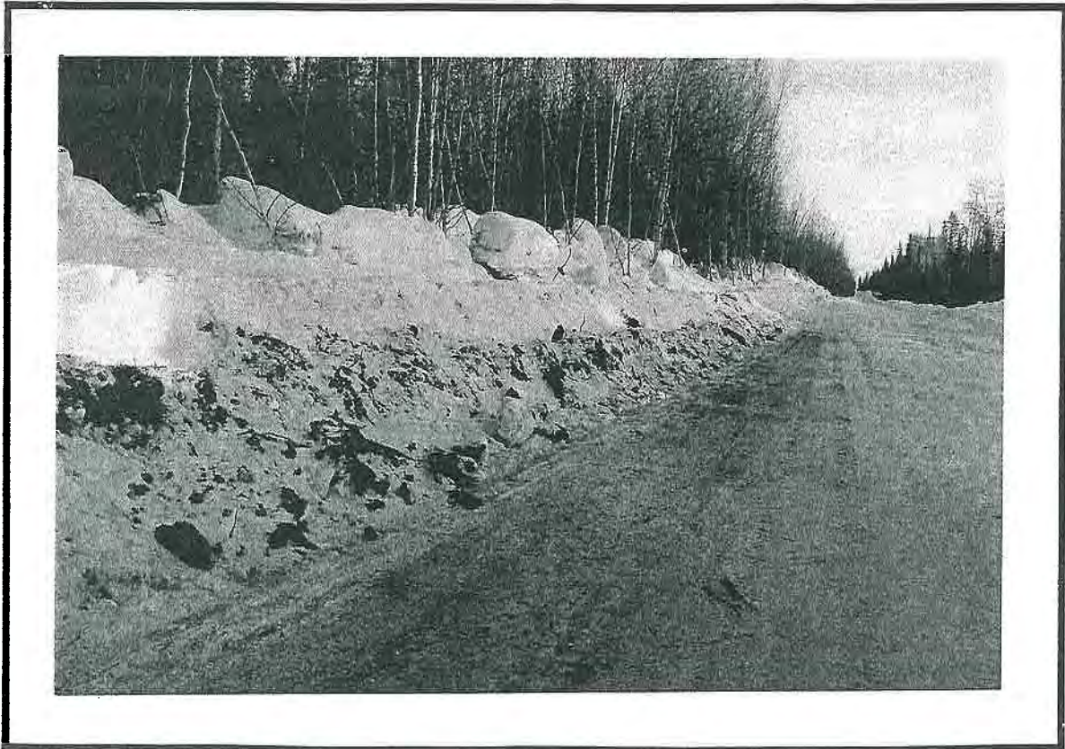
Dark Road Surface Together With Mineral Soil And Organics In The Windrow Indicates Surface Damage Is Occurring.
