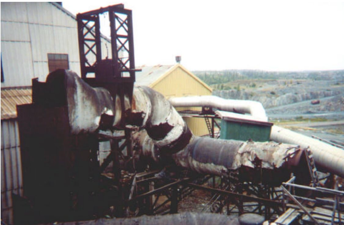
Photo #6: An old flue section that once connected the Cottrells to the stack (pre arsenic baghouse).
