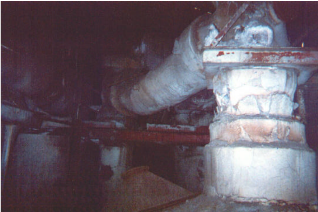
Photo #4: Exhaust flue from #2 roaster vessel to the dust collection cyclones. Note the white crystalline arsenic formation.
