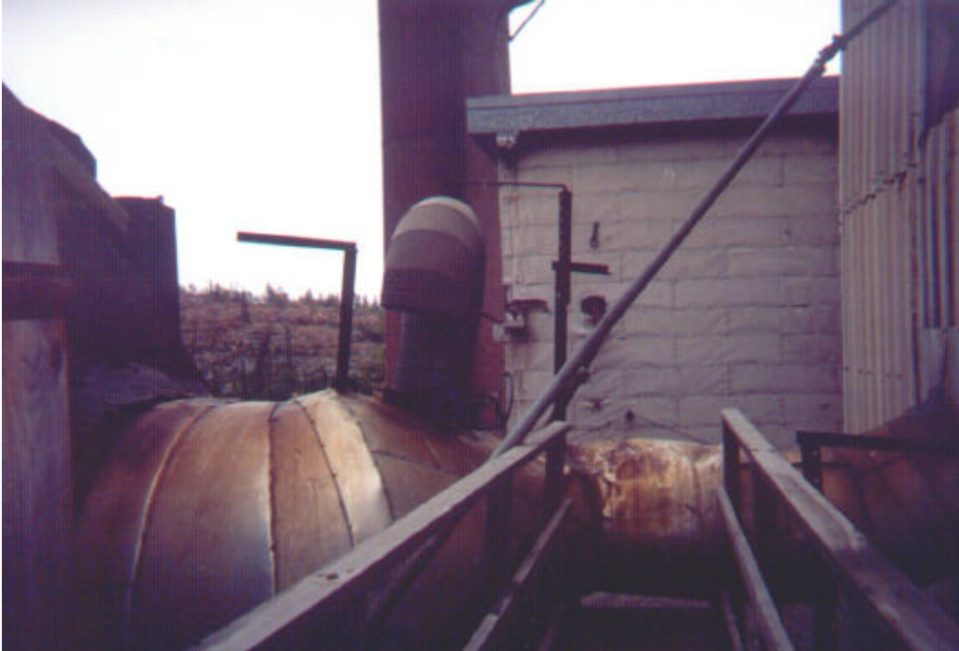
Photo #1: Transition section between roaster and Cottrell. Note change of diameter where the more recent flue replaced a section of much larger diameter old flue.
