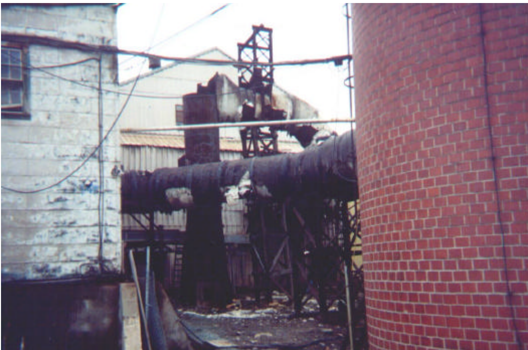
Photo #2: This view shows the base of the brick stack, the 40' high column, and the flue connecting the (no longer existing) AC roaster and the base of the stack.
