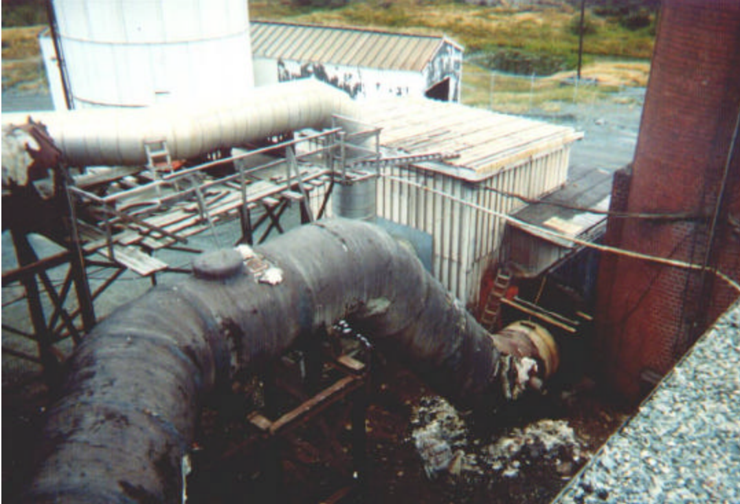
Photo #5: The black flue is direct from the AC roaster building to the base of the stack. The aluminum clad flue is quite recent, from the baghouse to the stack fan inlet.
